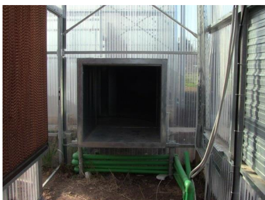
Picture 2. The lobby (wet pad on the left, blinds of fresh air on the right, the end point of the outside duct of the water/air recycling unit in the center, the 4 green pipes of the 2 heat exchangers)
