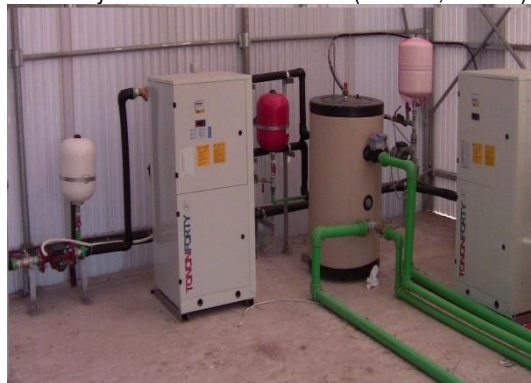
Picture 1. Heat pumps, tank of inertia and dilatation tanks of the water circuit, installed in the Engine room. Except the metal pipes, the special pipes (green colored) of PVC (Diam. 60 mm) of water recycling unit can be seen.
